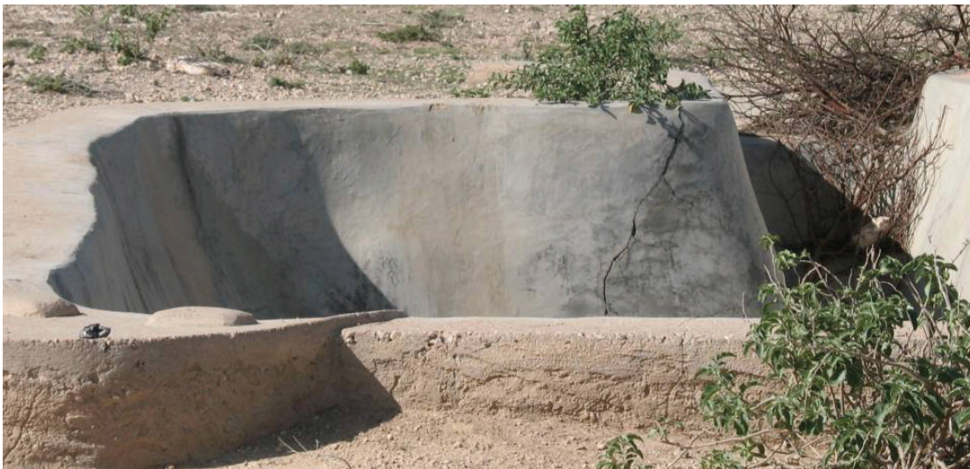
Figure 4.2 Cracks on berkad wall
