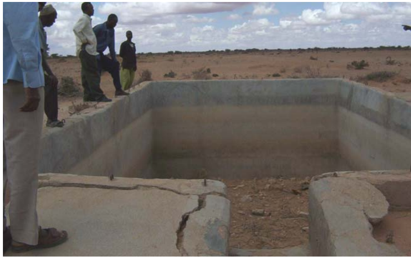
Plate 11: Cracking of a berkad
