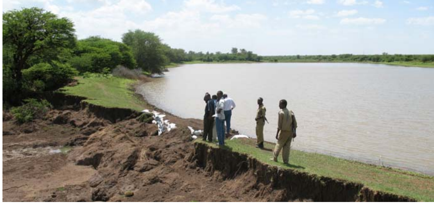
Plate 7: A section of a valley embankment destroyed by 2007 Gu rains
