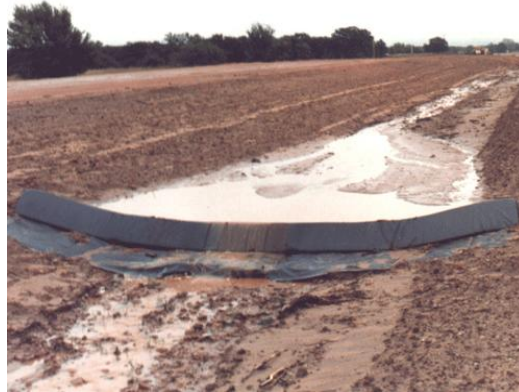
Figure 15: Small check dam on a relatively plain area in an erosion gully
