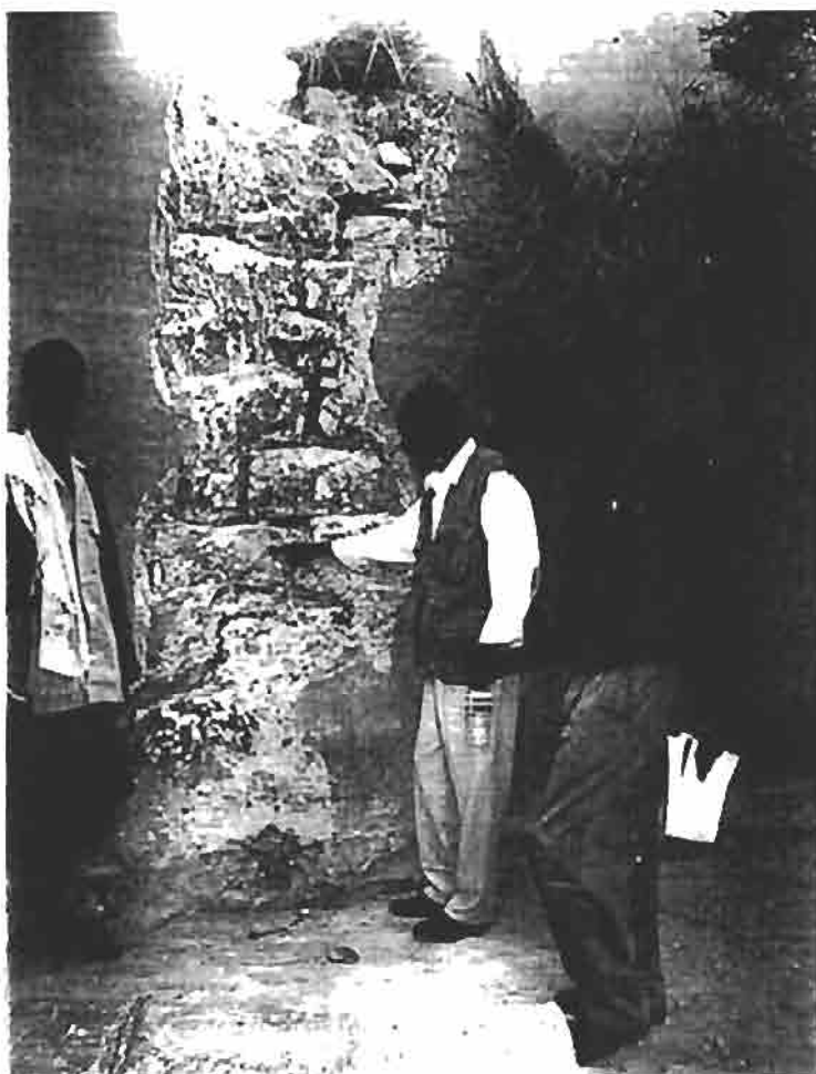
Plate 4: Cracks on berkad, Dhaxan village, Gardo District
